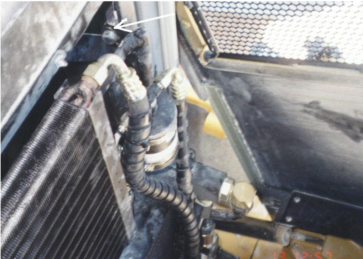
View of top right bracket with bolt indicated by arrow.
